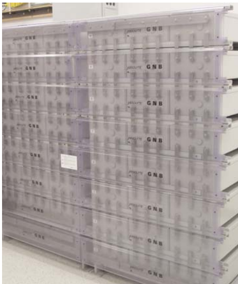
Power supplies are some of the most critical equipment you need to monitor.
